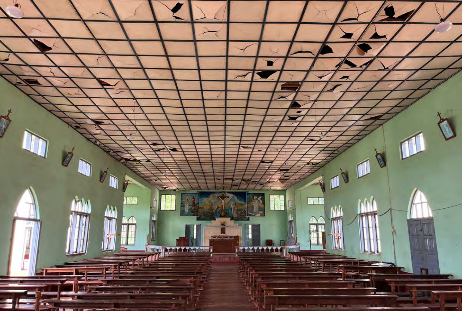
During a visit to Our Lady of Fatima Church, Amnesty International researchers surveyed the extensive damage it sustained due to a March 2022 Myanmar military air strike, 27 June 2022. © Amnesty International
