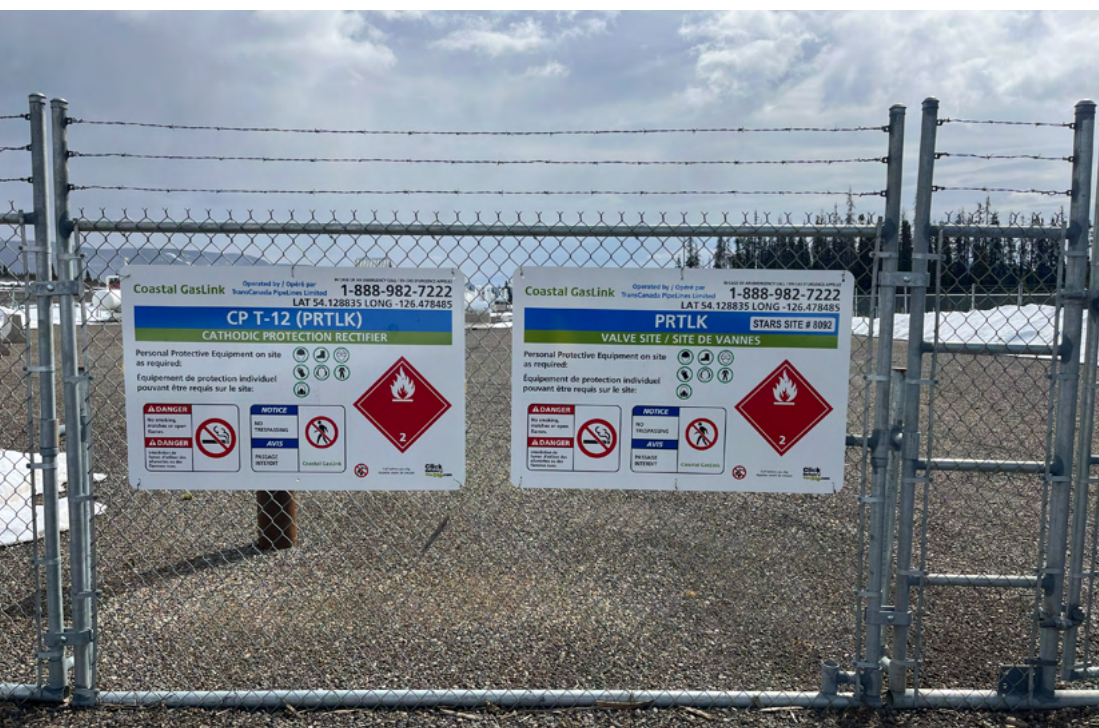
Valve station at the site of the planned Parrott Lakes compressor station, April 2025 © Amnesty International (photographer: Alli McCracken)
