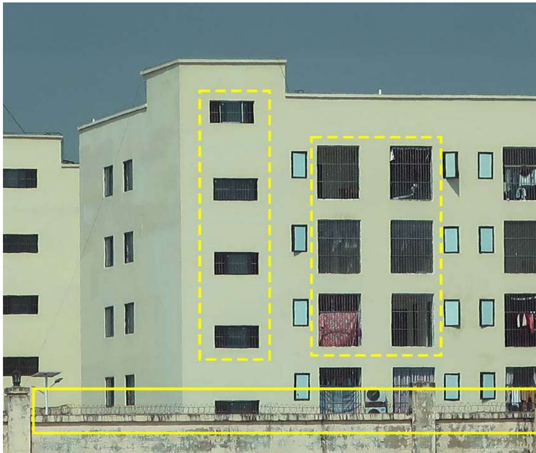
PP09: caged windows and barbed or razor wire on internal walls. © Amnesty International, 2024.
