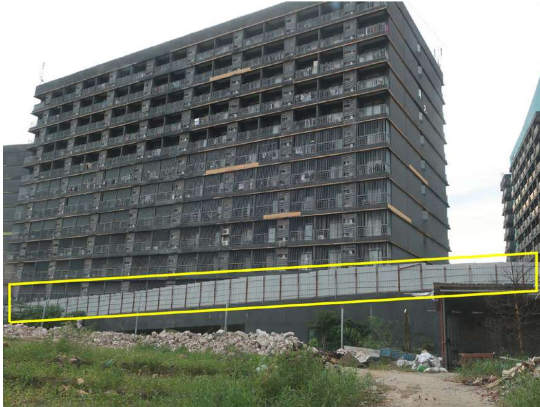
SI08: high perimeter walls that have been extended to make them higher using sheet metal. © Amnesty International, 2024.
